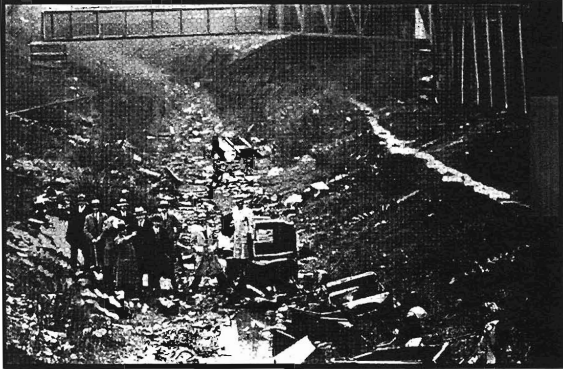
Excavations for the City Subway in former Morris Canal bed in Newark in the 1930s.
