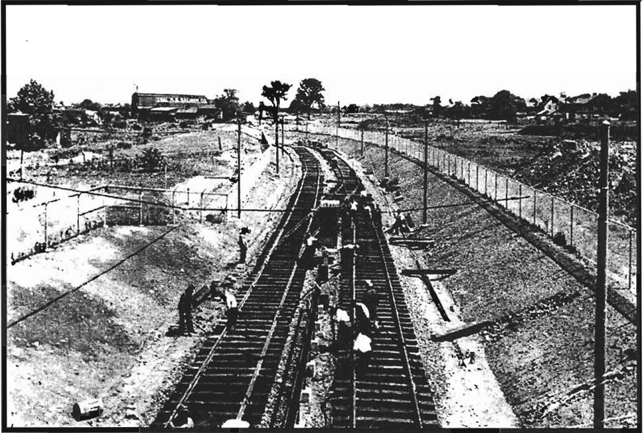
City railway under construction in 1934. View is looking north from Heller Parkway with H.B. Salmon building again shown on the west side of the former canal (courtesy of NJT).
