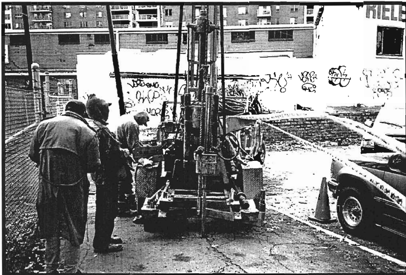
Soil boring (S-15A or S-15B) being drilled north of Franklin Avenue loop on November 10, 1995. View is looking west.
